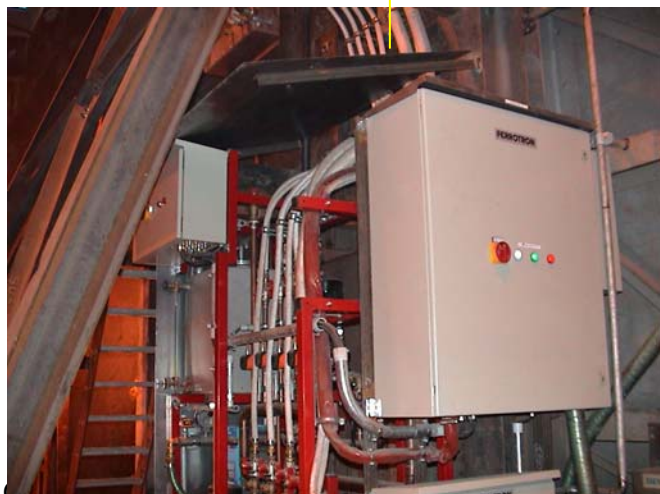
Control and cooling unit
